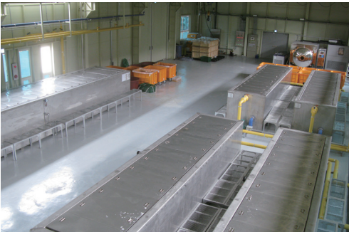
6. Consolidation facility, Taeon
